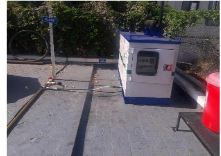
Use of Bio-methane for electricity generation
