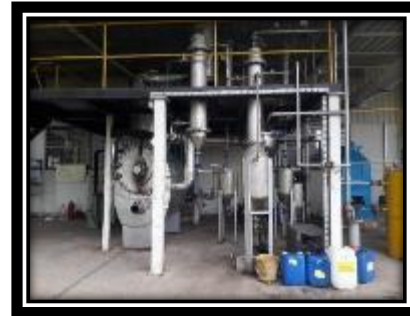
Installed and commissioned “Waste plastic to Fuel Conversion plant” with a yield of almost 70%.
